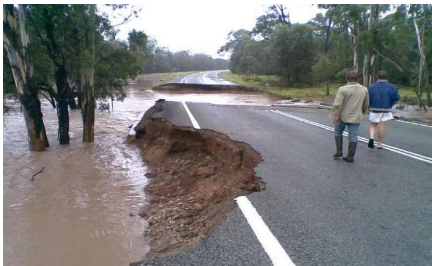
Figure 3- Flood damage to roads interrupting the produce supply
